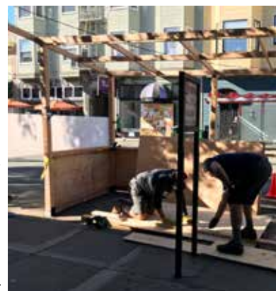
Coming a little late to the game, Kezar Bar and Restaurant constructed a parklet parallel to its frontage and half that of Val de Cole.
