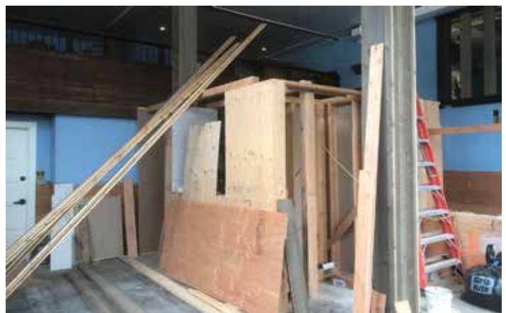
Anyone taking a peek through the door can see that a full-scale remodel is in progress—far from the original configuration of the old Ironwood restaurant of the last century. How long is our wait for the opening of the promised Blue Barn café? And does a sandwich shop duplicate nearby eateries?
