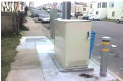
The AT&T boxes sit on a concrete platform and are surrounded by bollards that extend the original footprint by a third.
