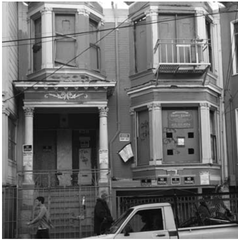
626-628 Cole Street has been derelict since a fire made it uninhabitable several years ago.
