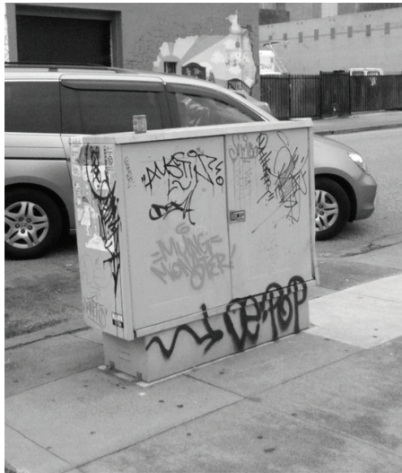
Permits for AT&T's 726 giant utility boxes are being processed neighborhood by neighborhood so that the cumulative effect will not be noticed.
