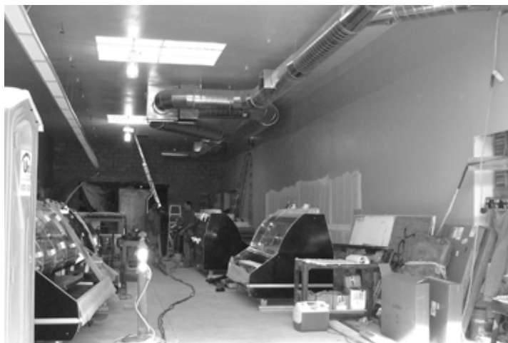
The adjacent building has been gutted, the back wall extended to the lot line and a mezzanine level added.
